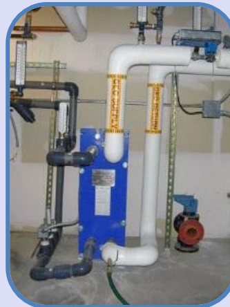
Ground source heat pump
