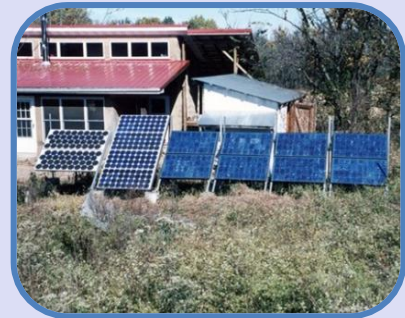
Solar panel ground installation
