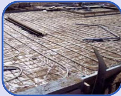
Photo Aldo Leopold Foundation, Leopold Legacy Center Construction Journal, Report 15.2—Mechanical Systems, www.aldoleopold.org
