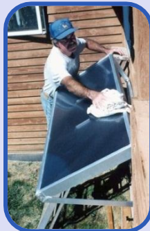
Solar heating panels
